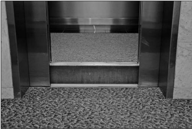
Figure 13-1: Platform not level with floor
