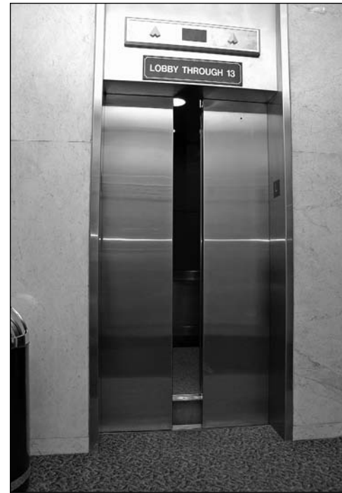
Figure 13-2: Elevator door not open fully
